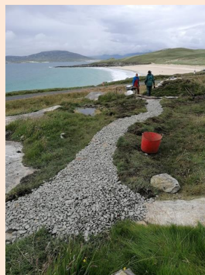
A section of new path was built from the West Harris Trust Talla na Mara centre to a drystone seat built by JMT volunteers last year
